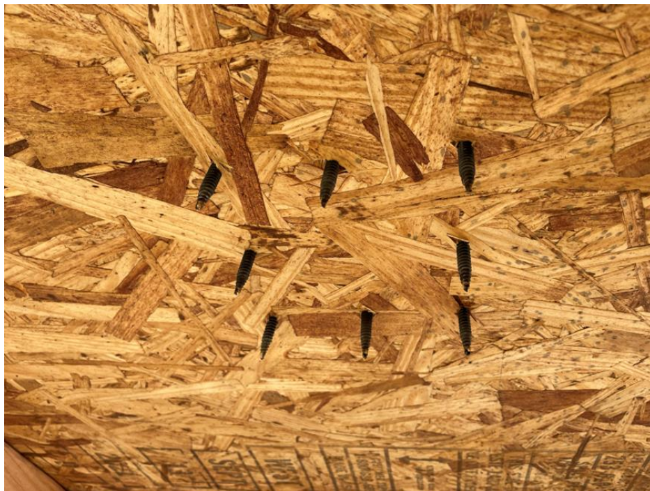
Photo No. 4 Underside of Test Desk After Test – no visible water penetration
