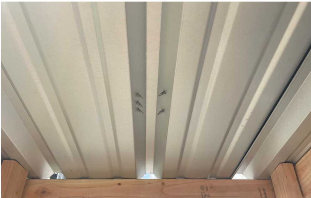
Photo No. 4 Underside of Test Desk After Test – no visible water penetration
