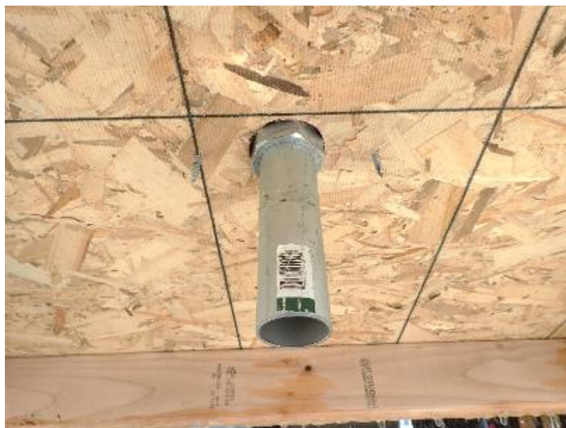
Photo No. 6 Underside of Test Desk After Test – no visible water penetration
