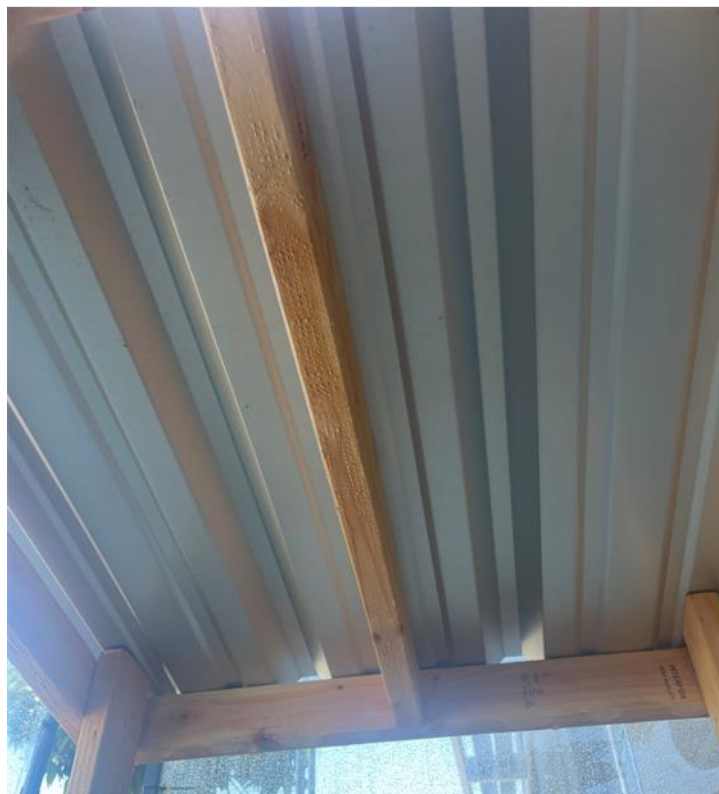
Photo No. 4 Underside of Test Desk After Test – no visible water penetration
