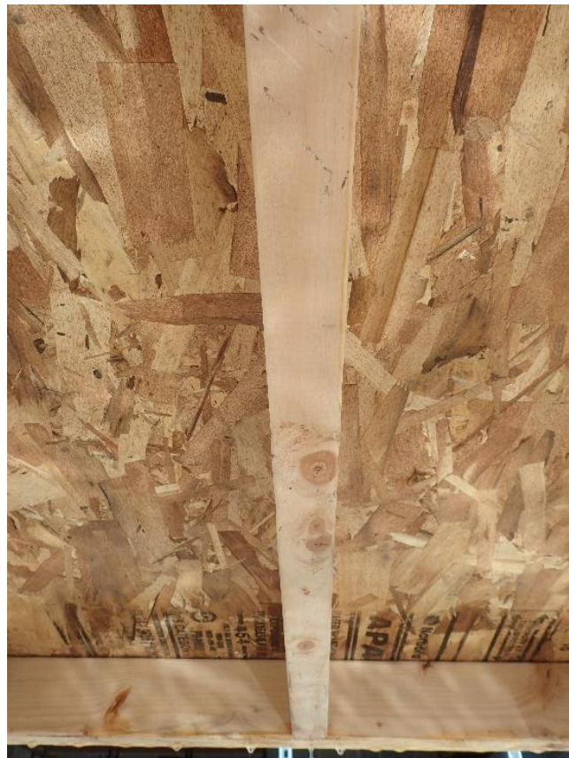
Photo No. 4 Underside of Test Desk After Test – no visible water penetration
